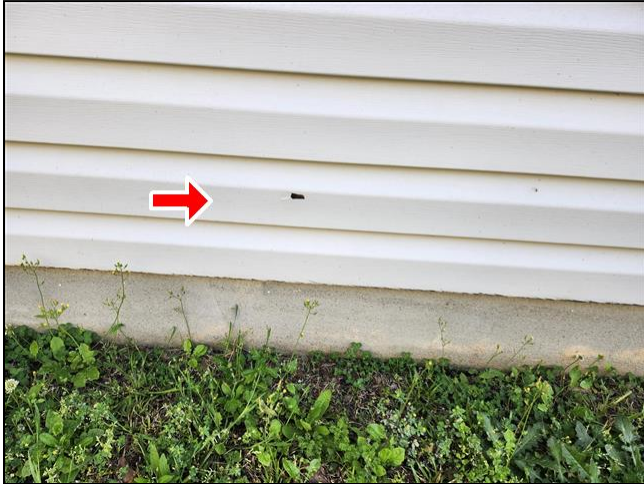
2.6 Item 1 (Picture) Area1 with hole
