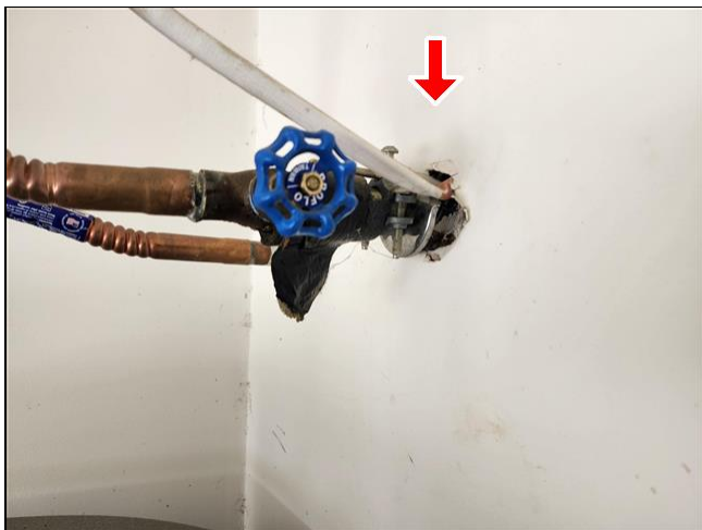
7.2 Item 1 (Picture) Electrical wire at water heater supply line.
