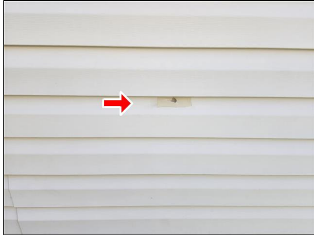
2.6 Item 2 (Picture) Area 2 with hole covered with tape
