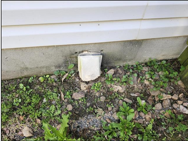
2.0 Item 1 (Picture) Damaged and blocked dryer vent cover
