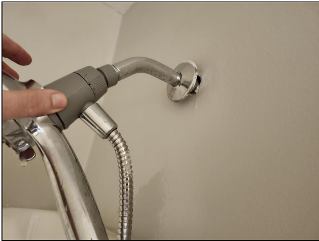
6.1 Item 1 (Picture) Loose shower head
