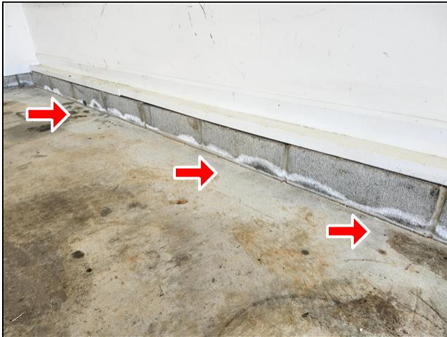
3.1 Item 1 (Picture) Efflorescence on concrete blocks in garage
