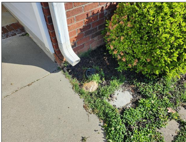
1.3 Item 2 (Picture) Recommend adding a downspout extension
