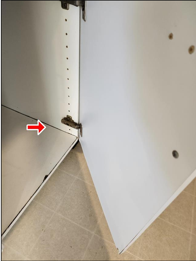
4.4 Item 1 (Picture) Kitchen cabinet door is loose at hinge
