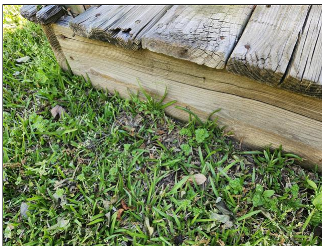
2.3 Item 2 (Picture) Deck in direct contact with soil
