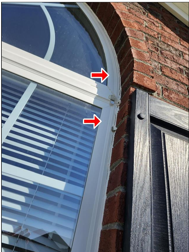
2.2 Item 1 (Picture) Cracked caulking.
