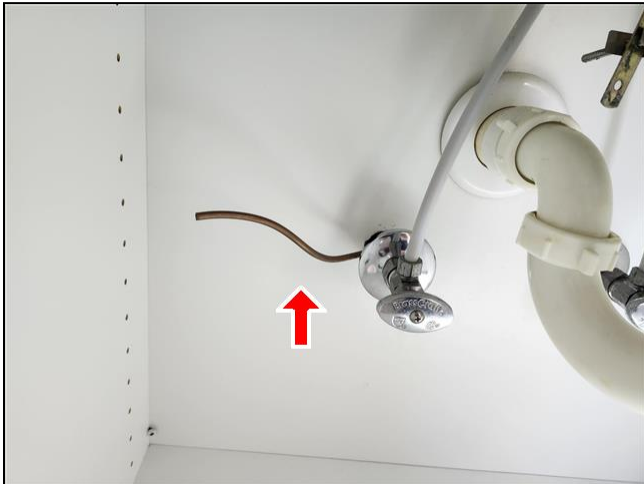
7.3 Item 1 (Picture) Ground wire under master bathroom sink (left side).
