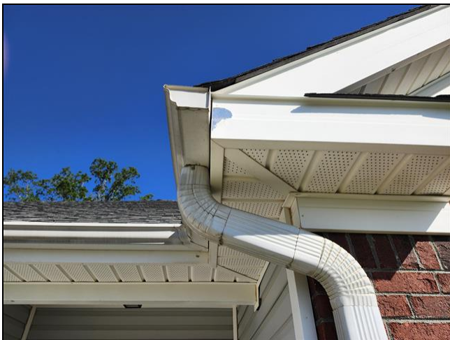
2.5 Item 1 (Picture) Peeled paint at eaves
