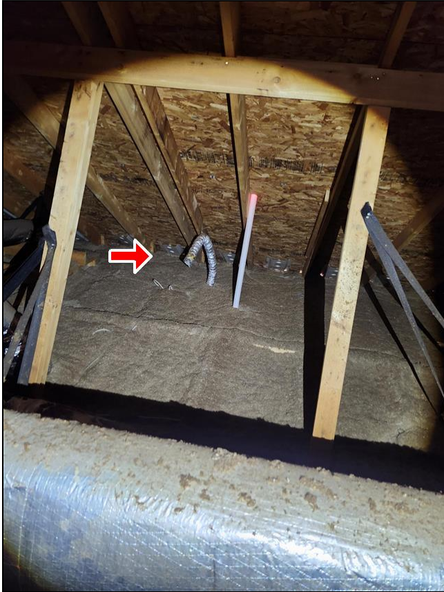
9.2 Item 1 (Picture) Bathroom vent terminates in the attic.
