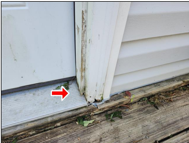
2.1 Item 1 (Picture) Exterior rear door trim moisture damage
