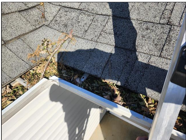
1.3 Item 1 (Picture) Gutter needs cleaned
