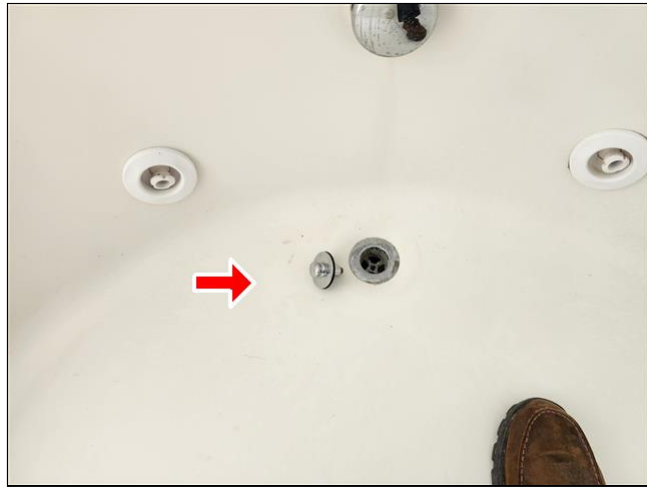
6.1 Item 2 (Picture) Drain stop is not attached.
