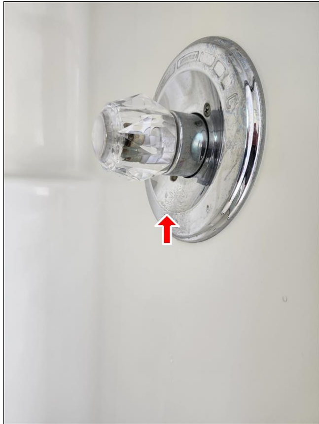
6.1 Item 4 (Picture) Leak at handle
