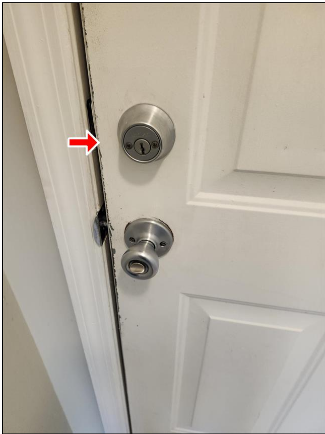
4.5 Item 1 (Picture) Double keyed deadbolts on garage door and rear exterior door.
